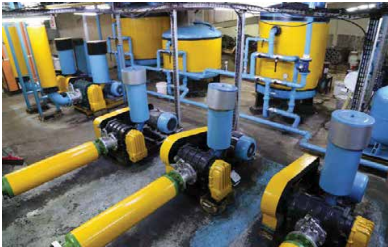
Pompa Blower Sewage Treatment Plant, Summarecon Mall Kelapa Gading
